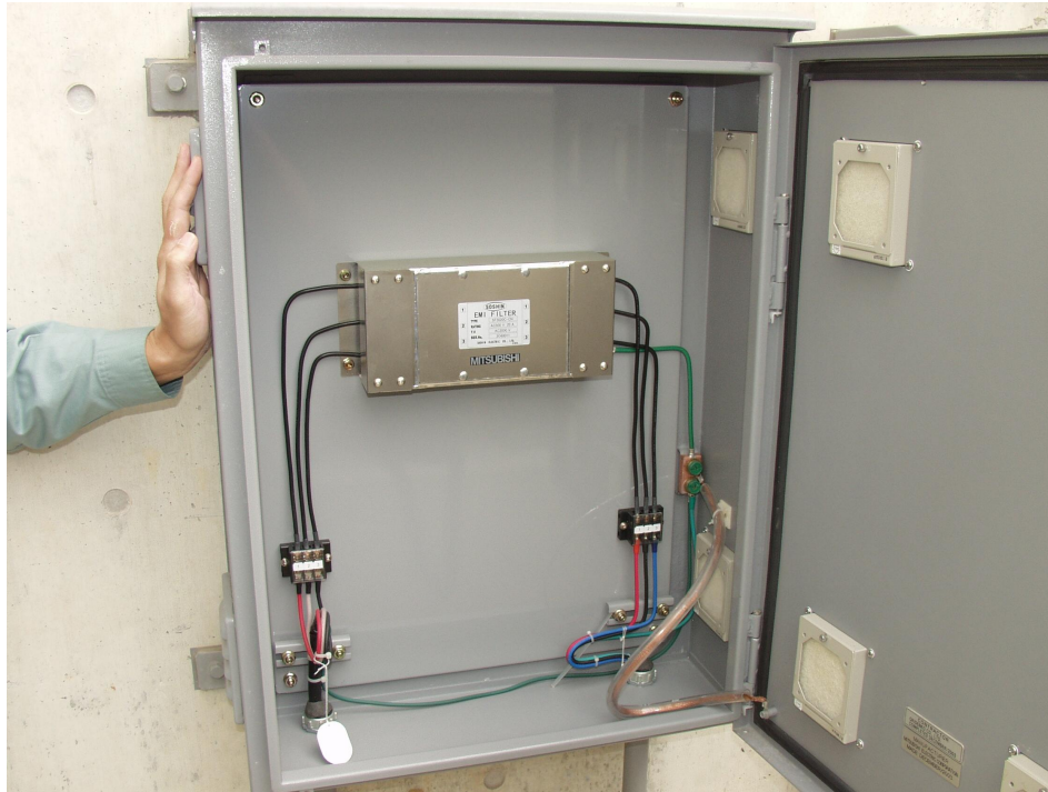
Figure 49 Improper Filter Configuration
