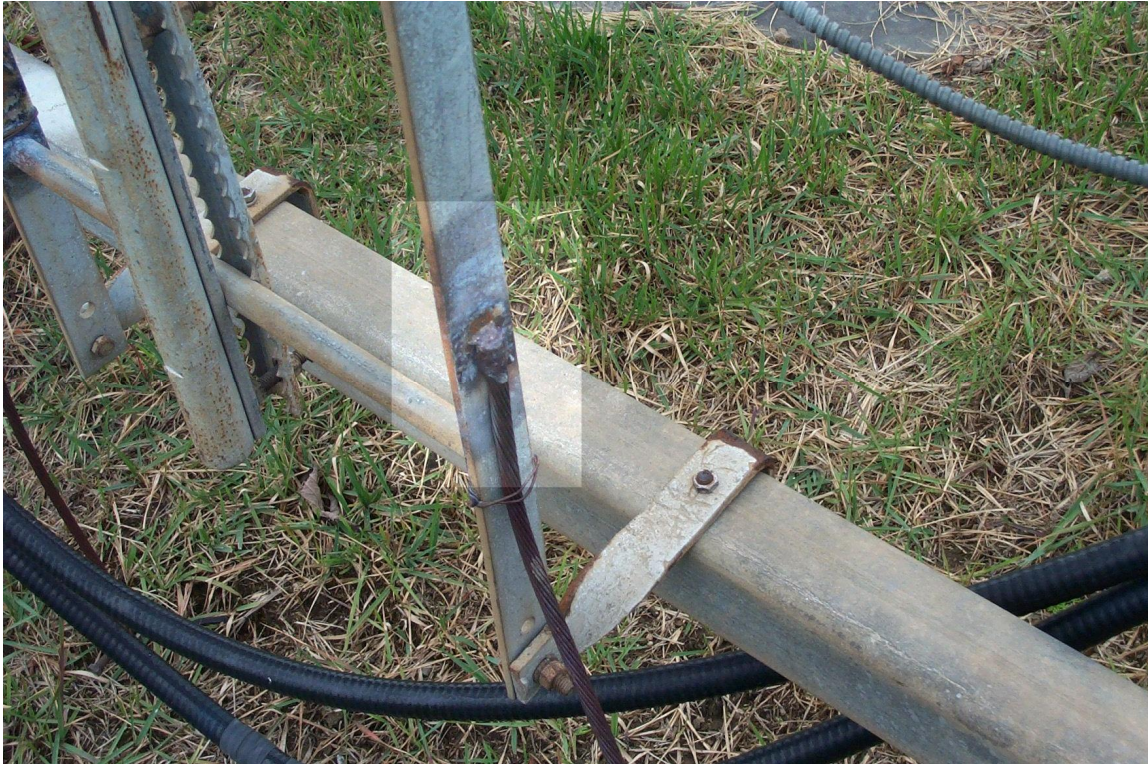
Figure 14 Ground Wire Welded to Galvanized Metal on Antenna Tower
