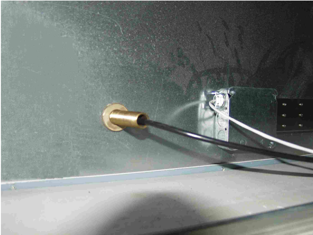
Figure 19 Coaxial Cable Penetration of a Shielded Room
