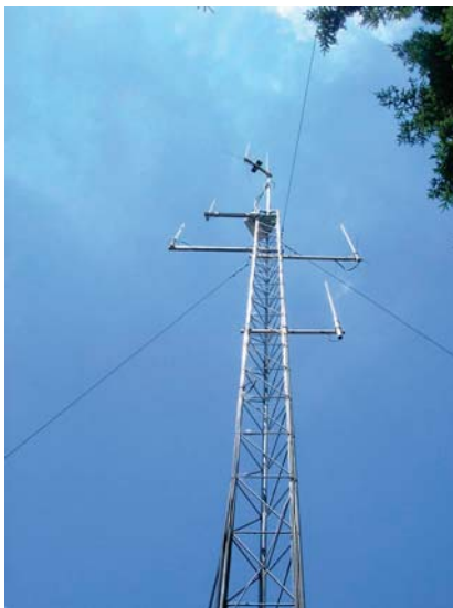
This tower supports the antennas for the KC7RJK repeater on 145.5 MHz in Eugene, Oregon. With these highly elevated antennas, the repeater enjoys wide coverage.
